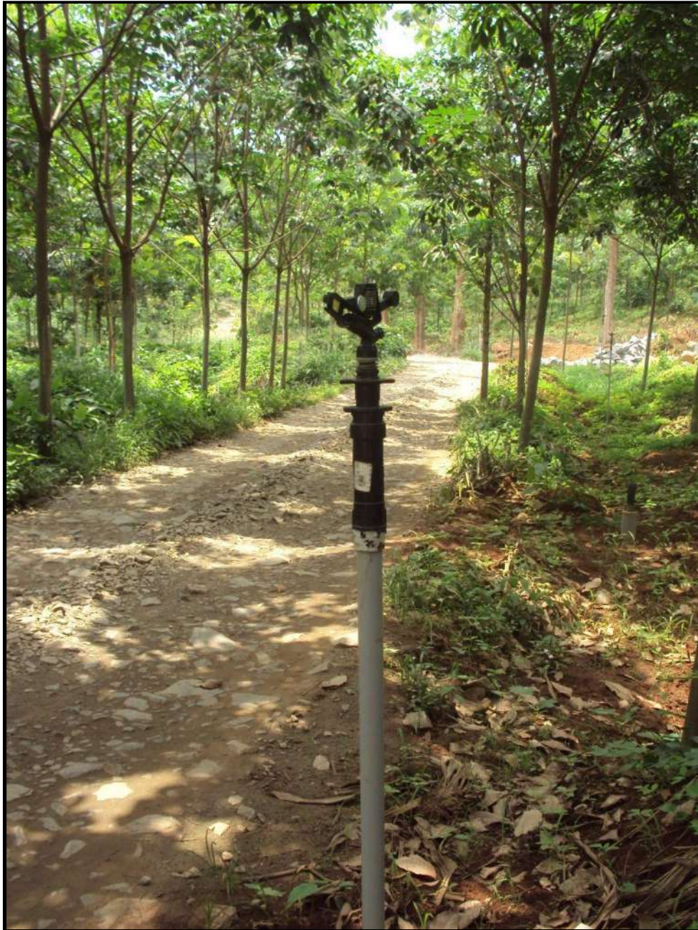
Photograph showing the fixed sprinklers installed along the roadside
