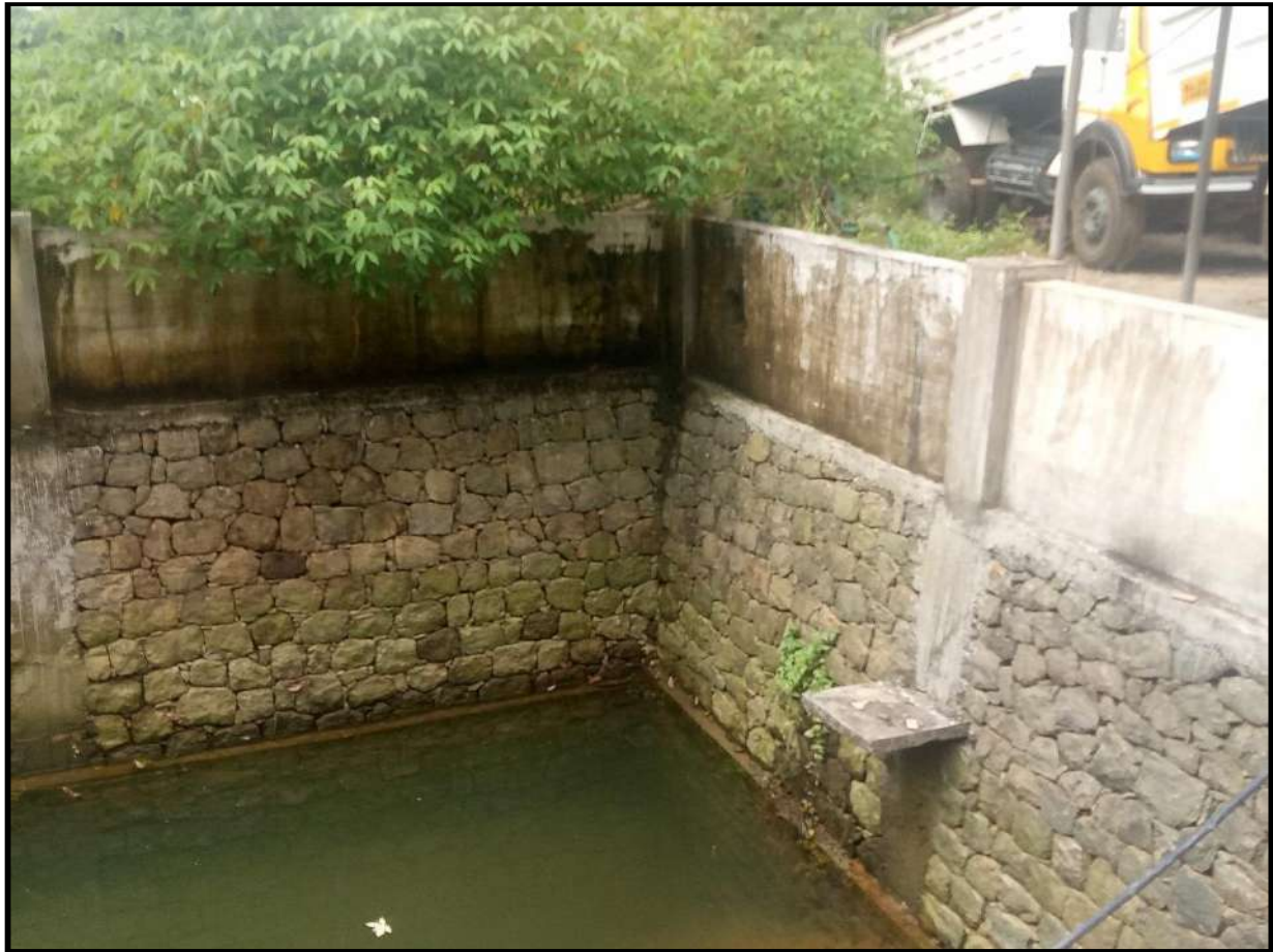
Photograph showing the rain water harvesting tank
